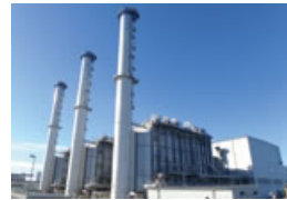
Ohgishima Power Station
