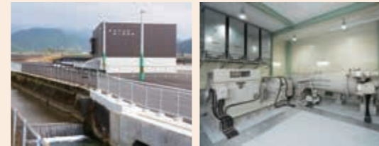
Hayatsuki River Shoreline No. 1 Power Station Horizontal axis cross-flow hydro-turbine and horizontal axis induction generator
