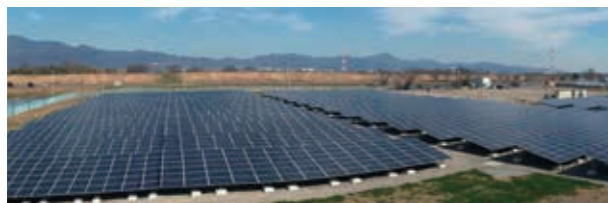
Solar power generation facility for Tokushima-shi No. 10 Water Purification Plant
