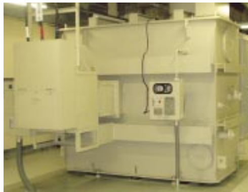
Transformer for Traction Substation
