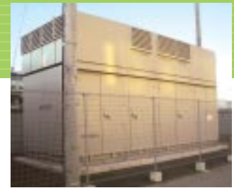
PCS for NAS Batteries
