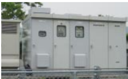
Braking Resistor Unit for Traction Substation
