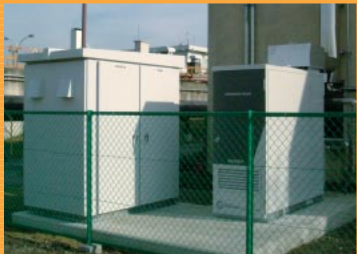
Biogas Generating System
