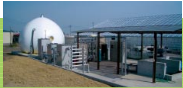
Biogas Power Generating System
