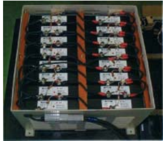
Fig. 1 External View of the Capacitor Modules
