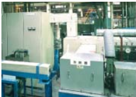
Wire material heating equipment
