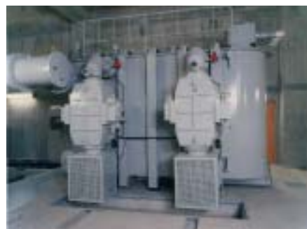
66kV 30MVA SF 6 gas-insulated transformer
