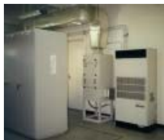
Corrosive gas removal facility
