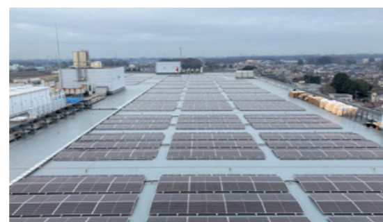
Solar power generation through on-site PPA on the roof of Isetan Mitsukoshi Logistics Center
