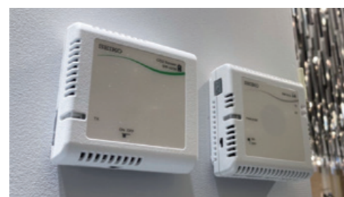
Environmental measurement sensors, Isetan Shinjuku Main Store Left: CO 2 sensor Right: Temperature and humidity sensor
