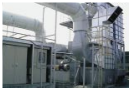
Deodorizing treatment equipment
