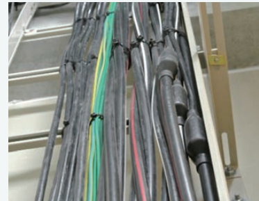
Ultralight Hybrid BH Cable installed
