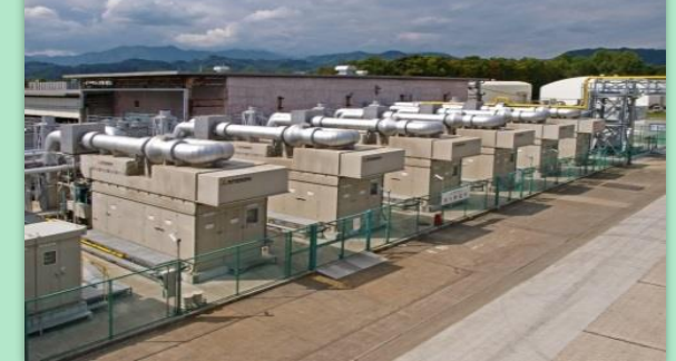
Gas Engine co-generation
