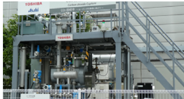
Experimental CO 2 Separation and Recovery Equipment
