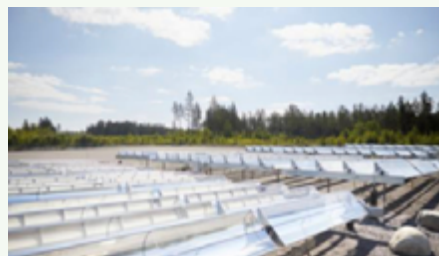
Solar collectors at Bari Brewery in Italy
