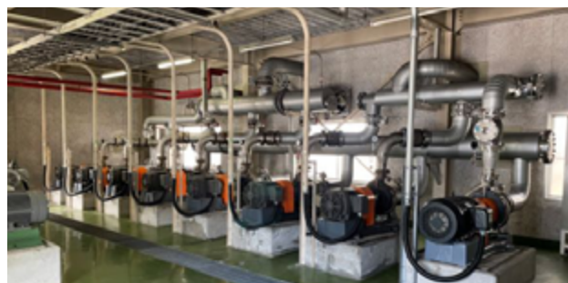
Water treatment facility (Nagoya Brewery)
