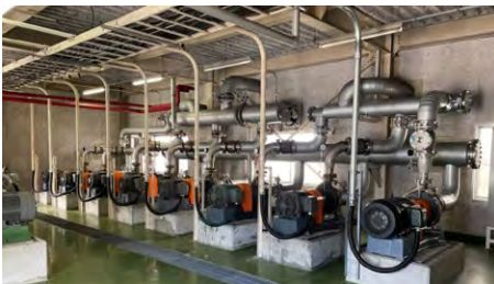
Water treatment facility (Nagoya Brewery)
