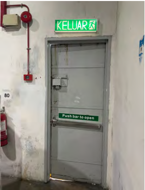
Push-locks installed on 14 emergency doors for a production site
