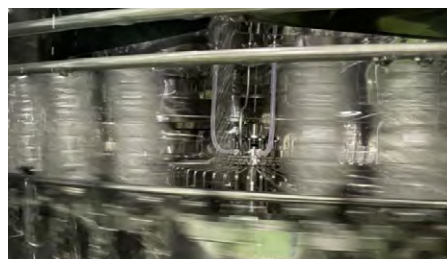
Water recovery and sterilization facilities (Akashi Plant in Japan)
