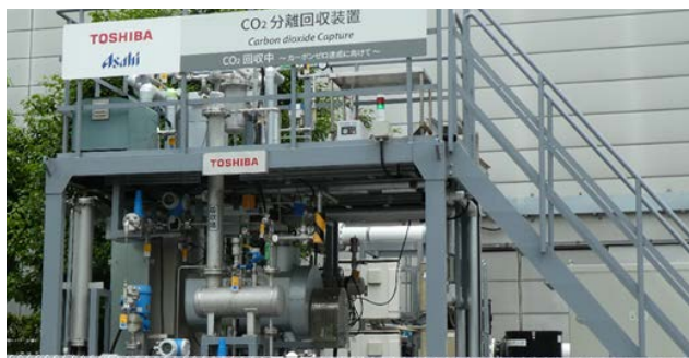
Experimental CO 2 Separation and Recovery Equipment
