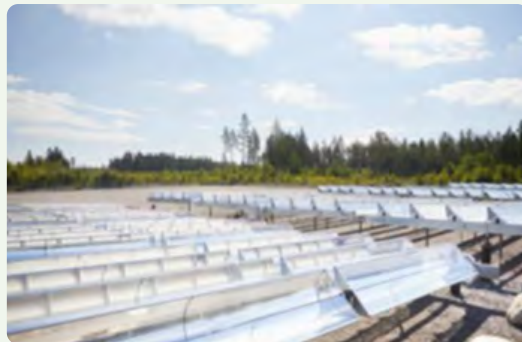
Installation of solar collectors at the Bari Brewery in Italy
